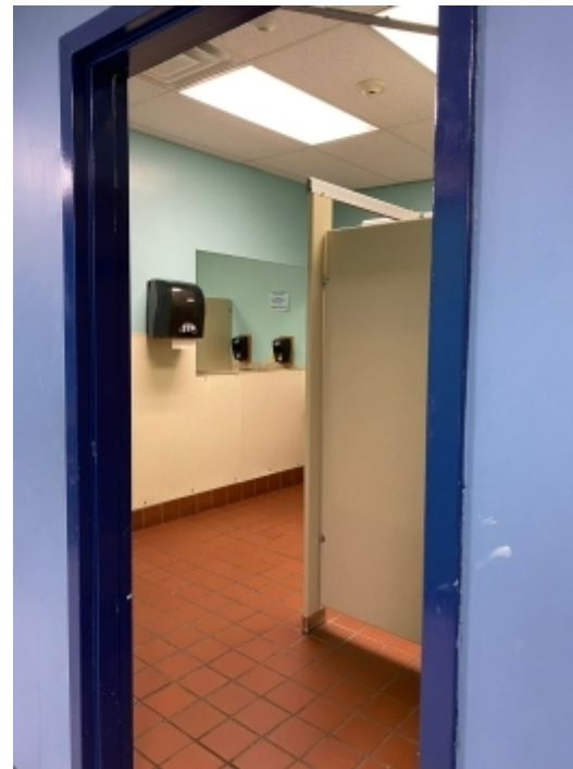
Northern bathroom plumbing routinely fails and needs to be replaced.
