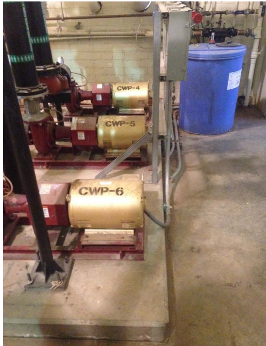
Condensing Water Pumps
