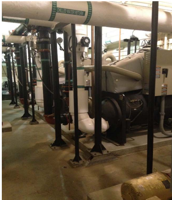
Central Cooling Plant
