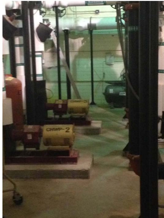
Chilled Water Pumps
