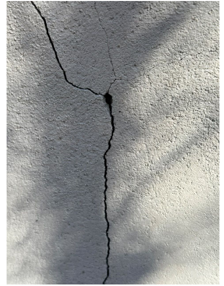
Figure 3: Detail View of Existing Stucco Cracking.
