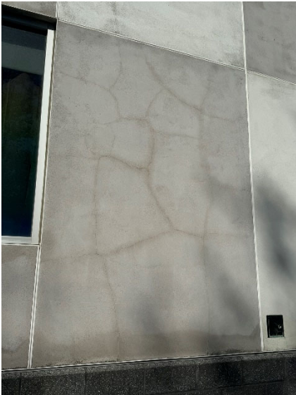
Figure 9: Detail View of East Elevation with Control Joints, Yet Excessive Cracking.
