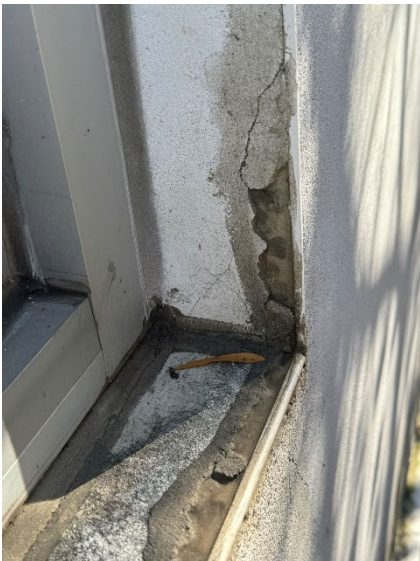
Figure 4: Detail View of Condition of First Floor Window Stucco Sill.
