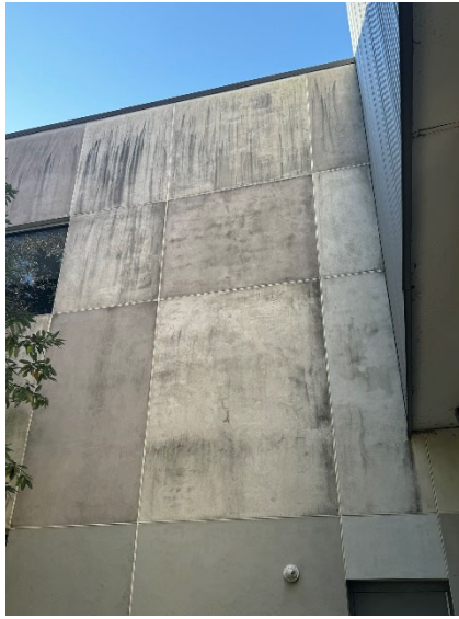
Figure 12: Detail View of North Elevation with Control Joints, Yet Excessive Cracking. Note Organic Growth Due to Excessing Stored Moisture.
