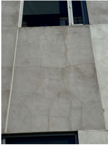
Figure 7: Detail View of South Elevation with Control Joints, Yet Excessive Cracking.
