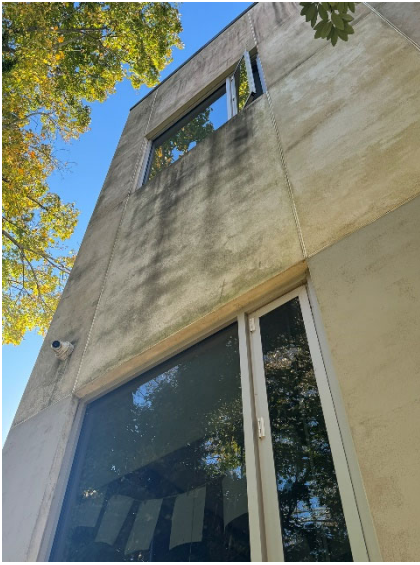
Figure 11: Detail View of North Elevation with Control Joints, Yet Excessive Cracking. Note Organic Growth Due to Excessing Stored Moisture.
