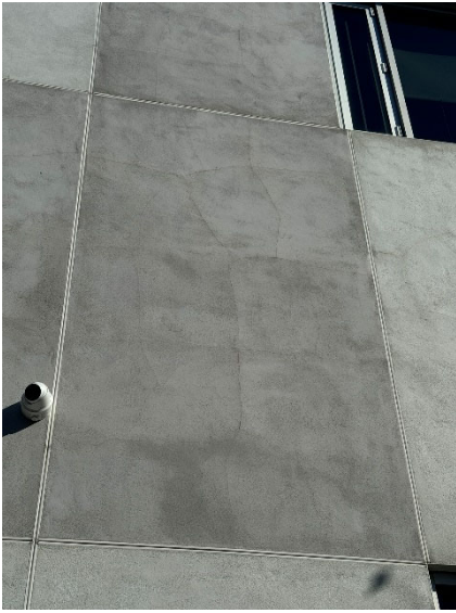
Figure 6: Detail View of South Elevation with Control Joints, Yet Excessive Cracking.
