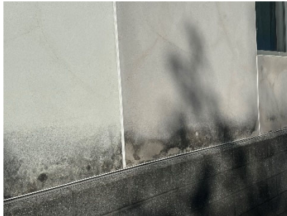
Figure 10: Detail View of East Elevation with Control Joints, Yet Excessive Cracking. Note Organic Growth Due to Excessing Stored Moisture.
