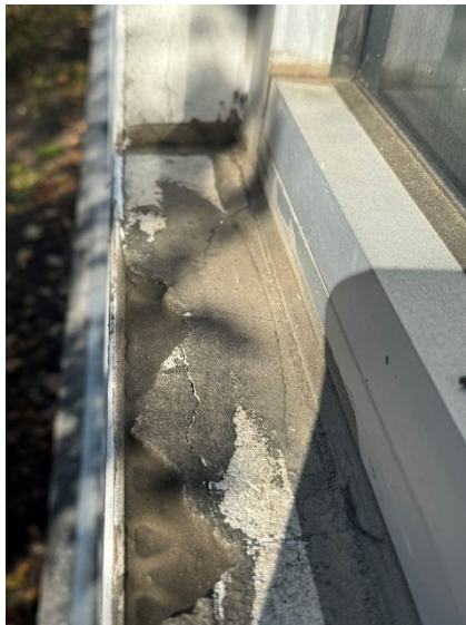
Figure 5: Detail View of Condition of First Floor Window Stucco Sill.
