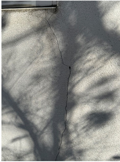
Figure 2: Detail View of Existing Stucco Cracking.
