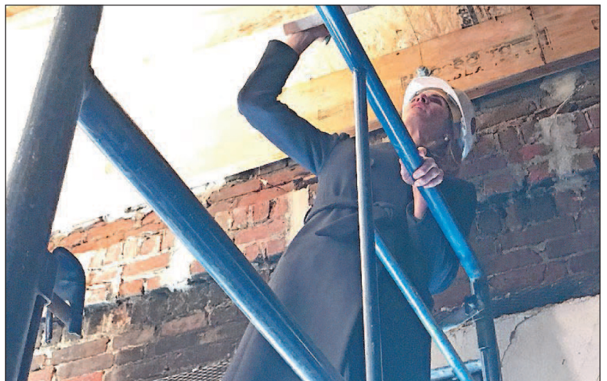
U.S. Rep. Trahan, D-Westford, who represents the 3rd Congressional District, signs a roof truss inside the former B.F. Brown School in Fitchburg. NewVue Communities is renovating the building into artist housing.
