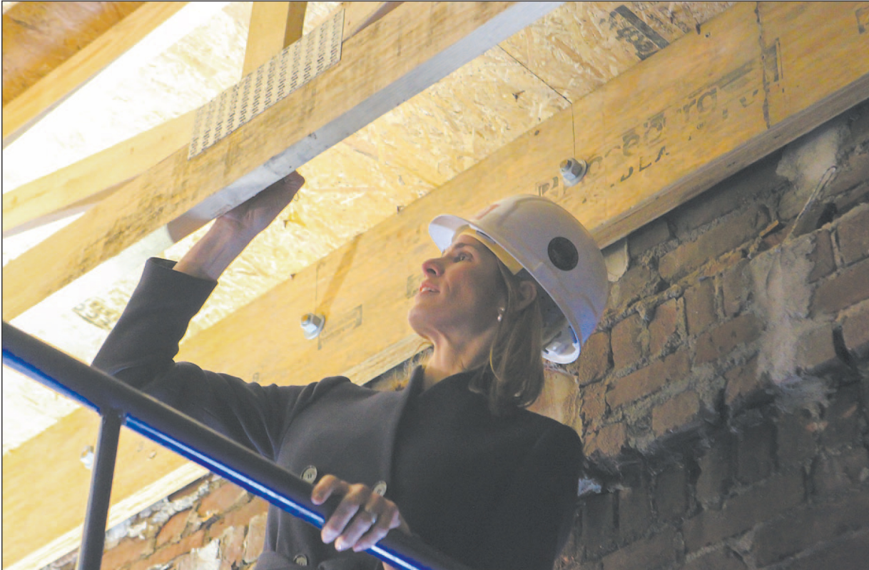
U.S. Rep. Lori Trahan signs her name on the wooden truss at the BF Brown School renovation, where other dignitaries had signed it at the start of the work on the site.
