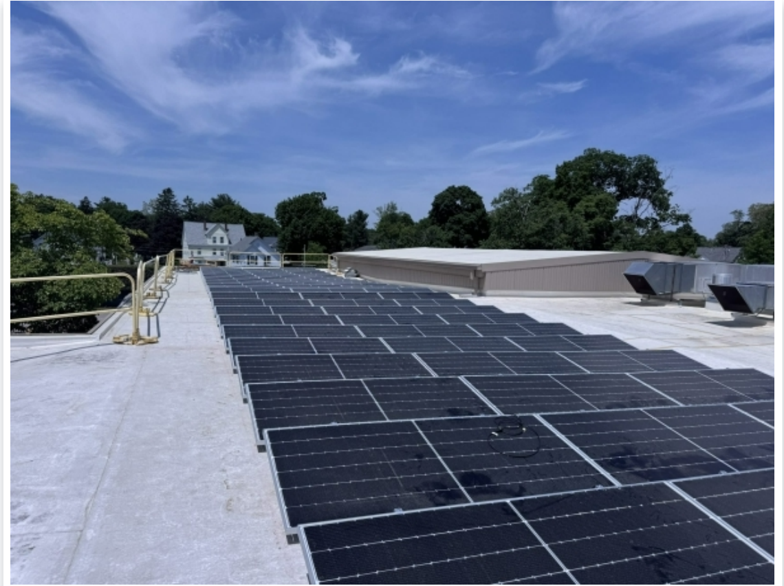
Installed array on the Middle School roof, June 5
