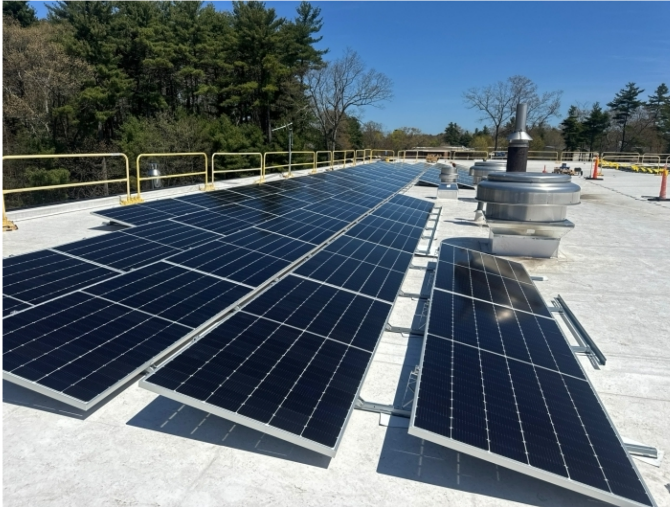
Photo reference: roof mounted panel arrays
