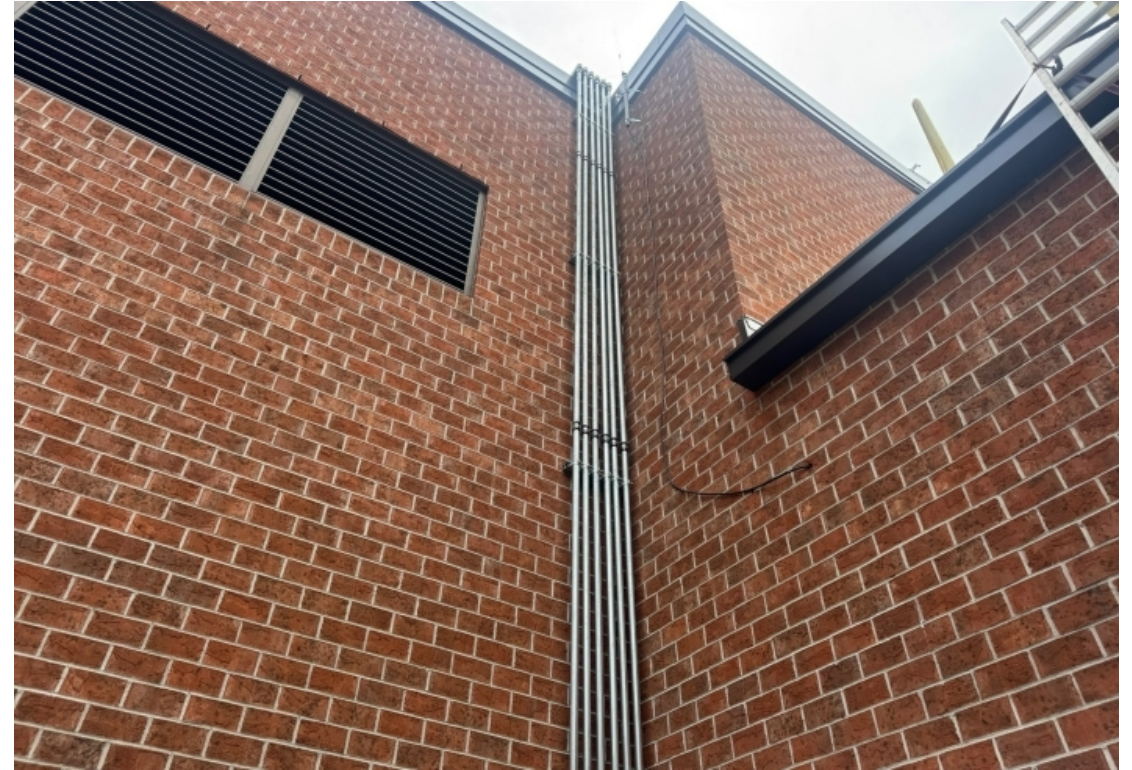
Exterior conduit routes supporting system connection
