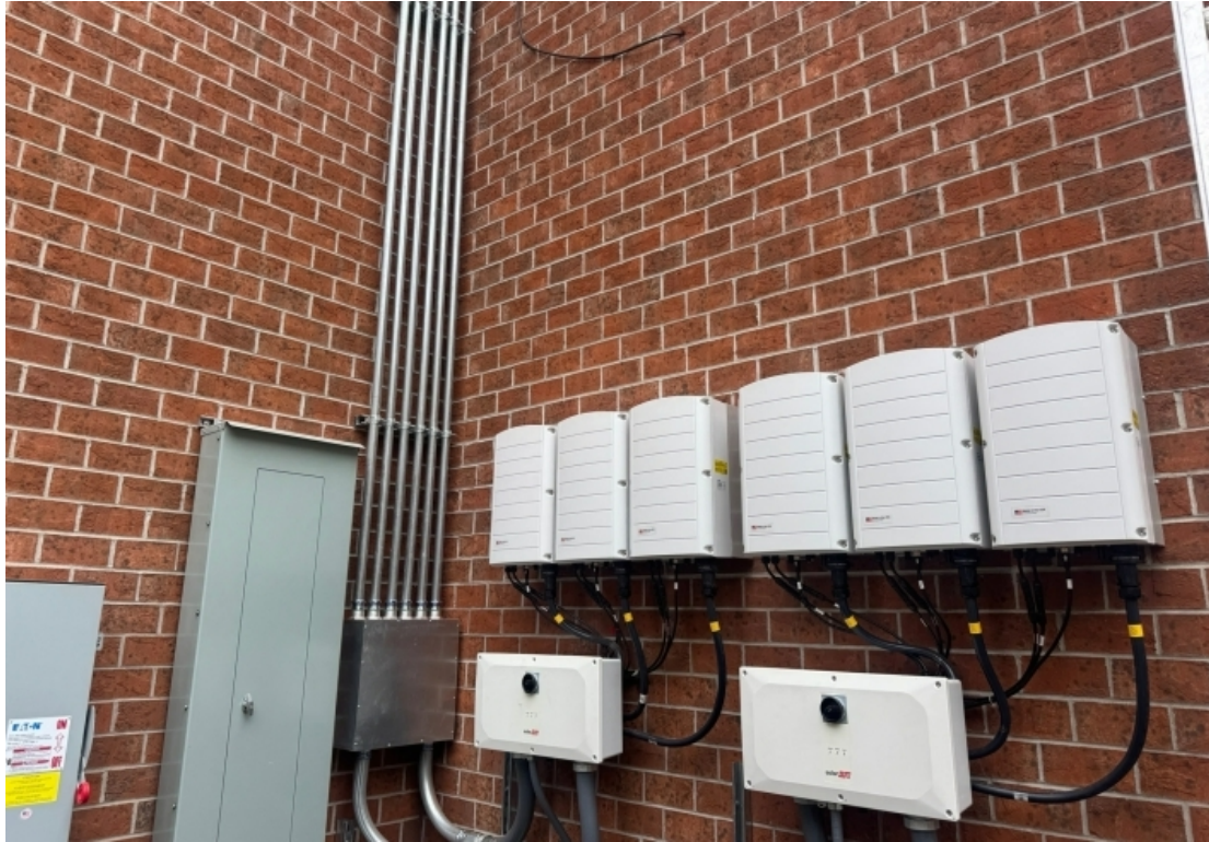
Mounted and wired electrical equipment near the loading dock
