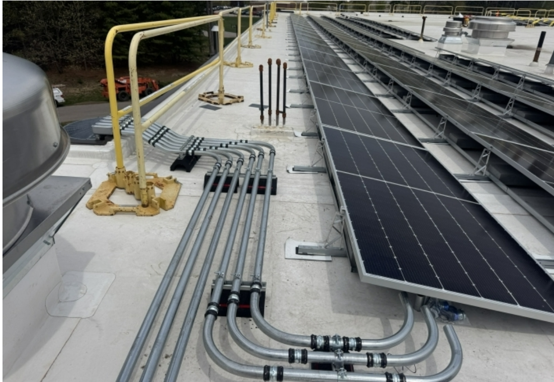
Conduit and wire routing on the roof
