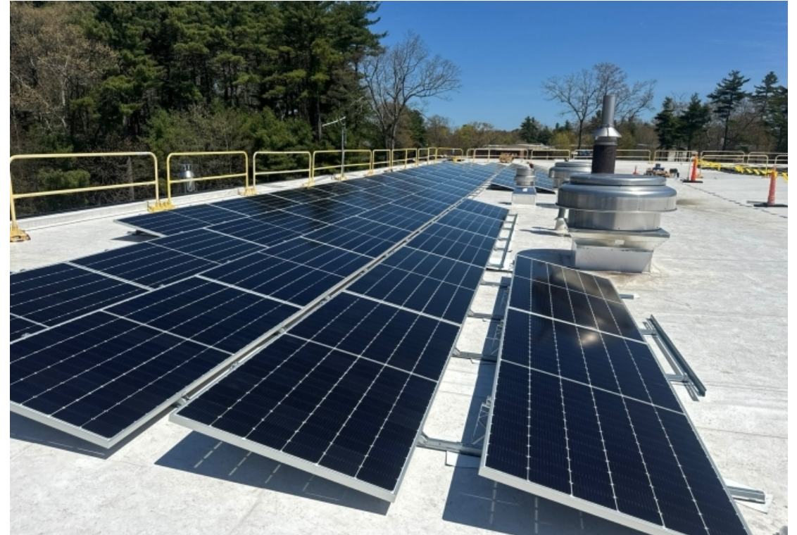
Installed panel arrays across the roof area
