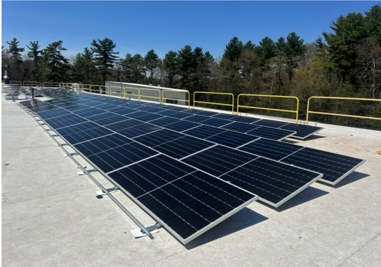
Roof mounted solar panels and racking in place
