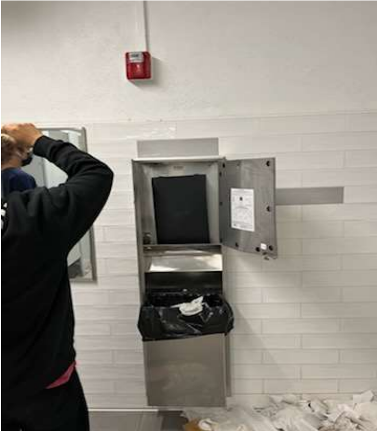
G-Bldg 1 st Floor Boys Rstroom - Has now been completely pulled off wall.
