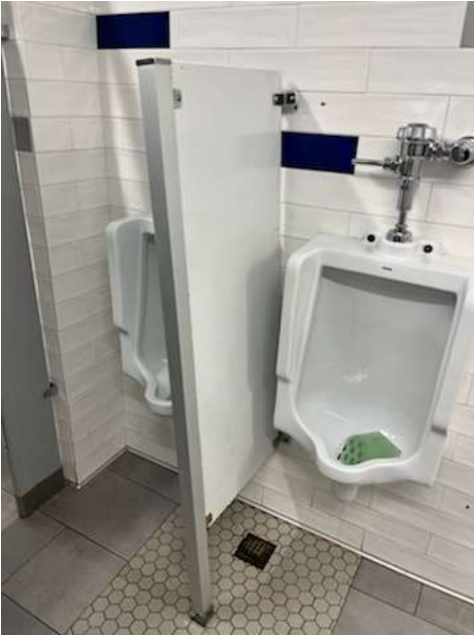
E-Bldg 1 st Floor Boys Restroom ..... These dividers now ripped off the wall
