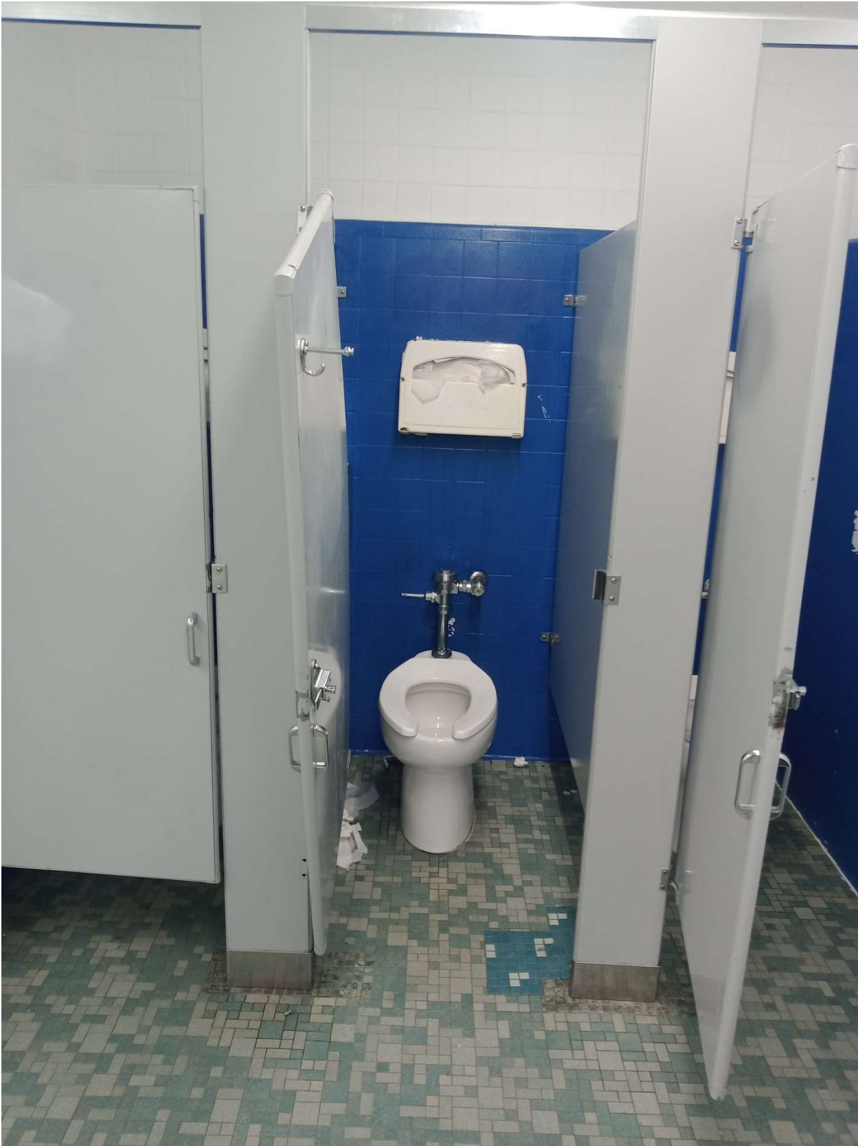
G-Bldg 2 nd Floor Boys Restroom .... Kicked-In Stall Door, broken off hinges.
