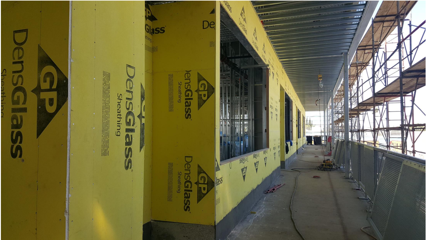
Exterior sheathing and walkway railing installation in progress at bldg C south.
