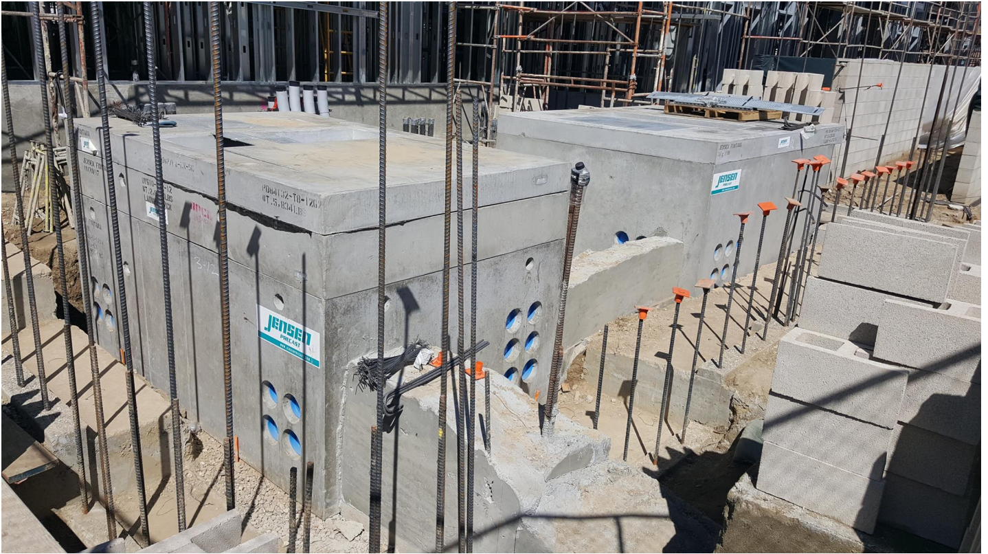
Transformer and Switch concrete vaults installation at the Electrical Yard. CMU wall installation at the electrical yard and utility yard in progress.
