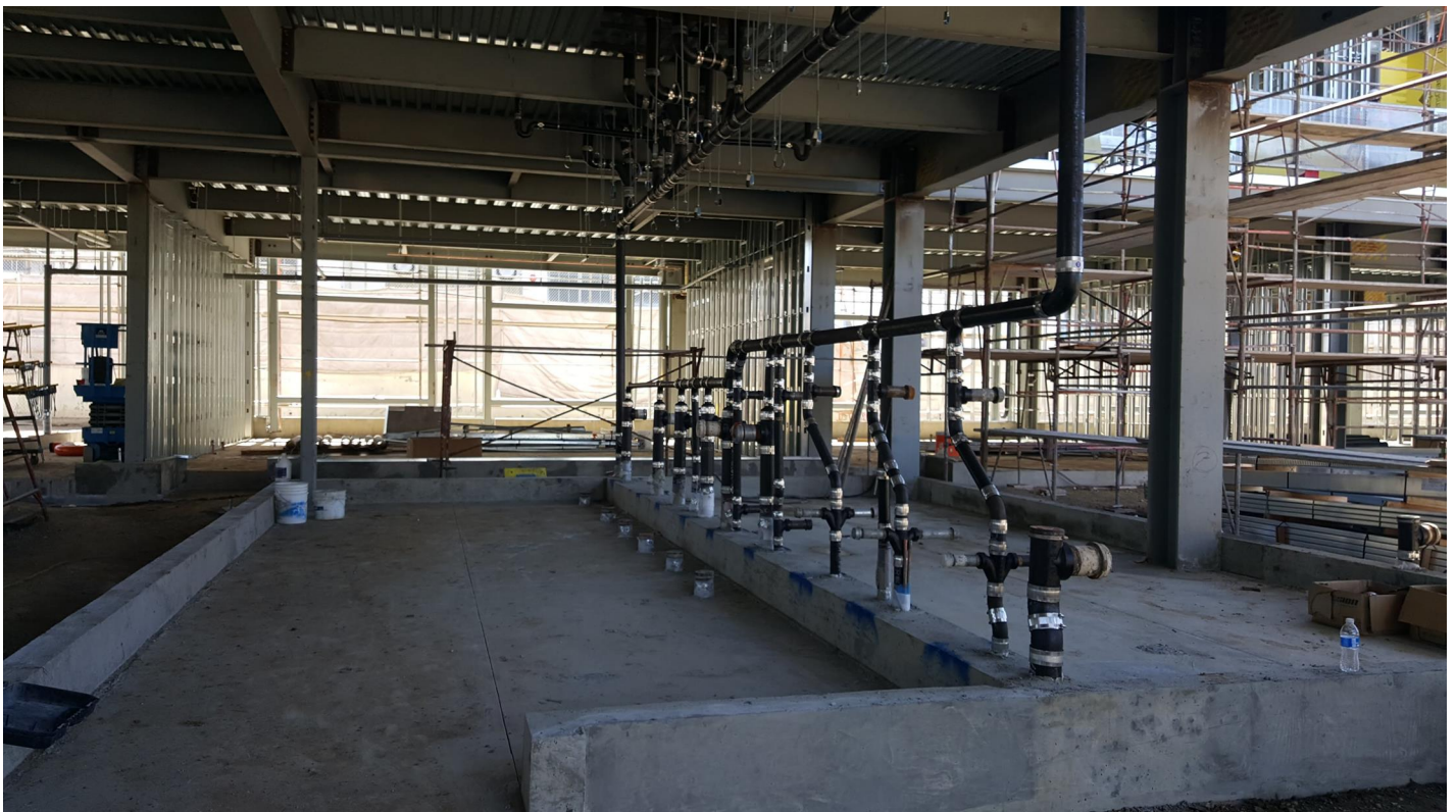
Installation of interior metal stud framing in progress at bldg C south, 1st floor. Installation of all MEP in progress at 1 st floor restrooms, bldg C.
