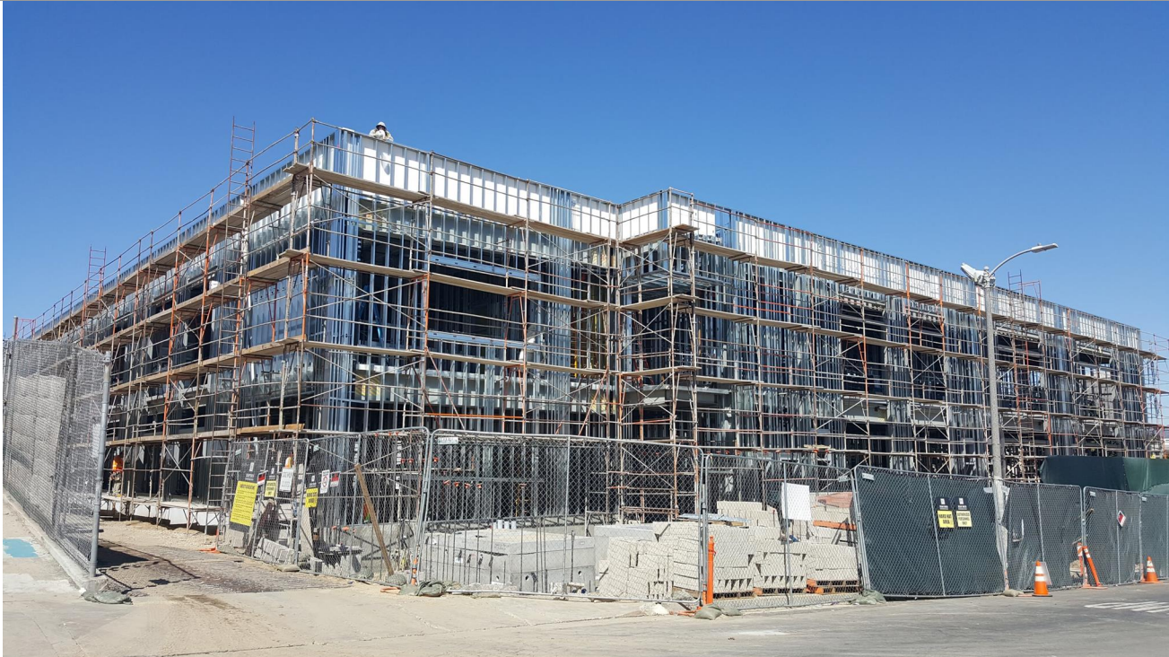
Installation of exterior and interior metal stud framing in progress at bldg. C south and east wing. Installation of transformer and switch concrete vaults at the electrical yard completed.
