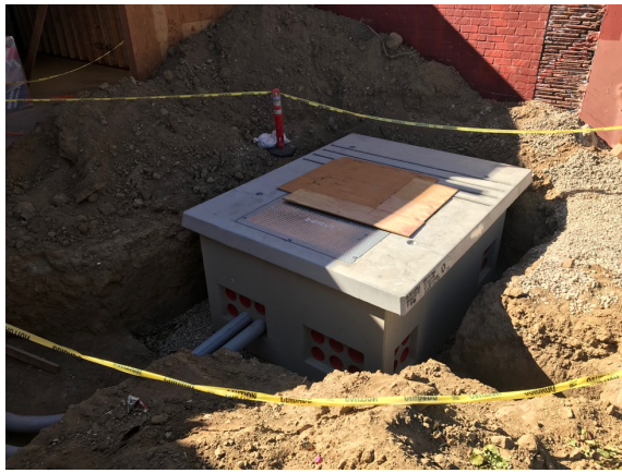
Utility Vault [1] off of Sherman Way
