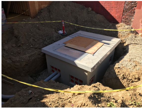
Utility Vault [1] off of Sherman Way
