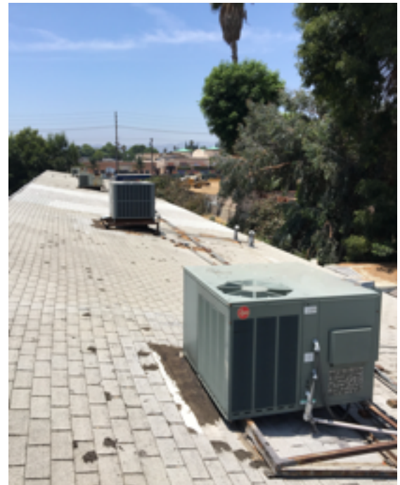
Figure 4: View of units on roof
