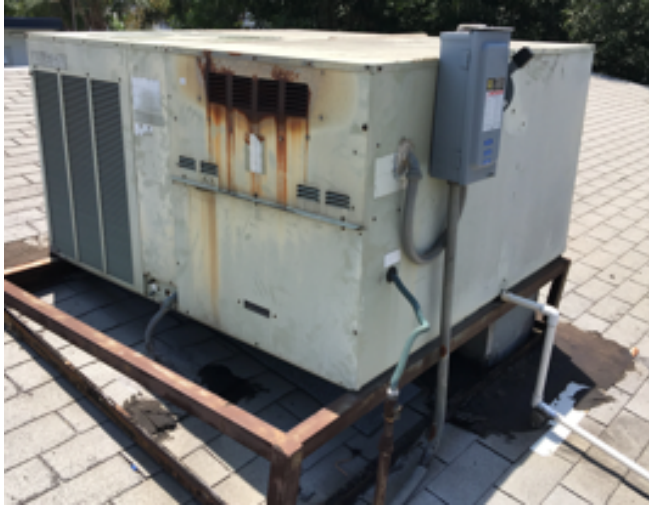
Figure 1: Photo of Unit
