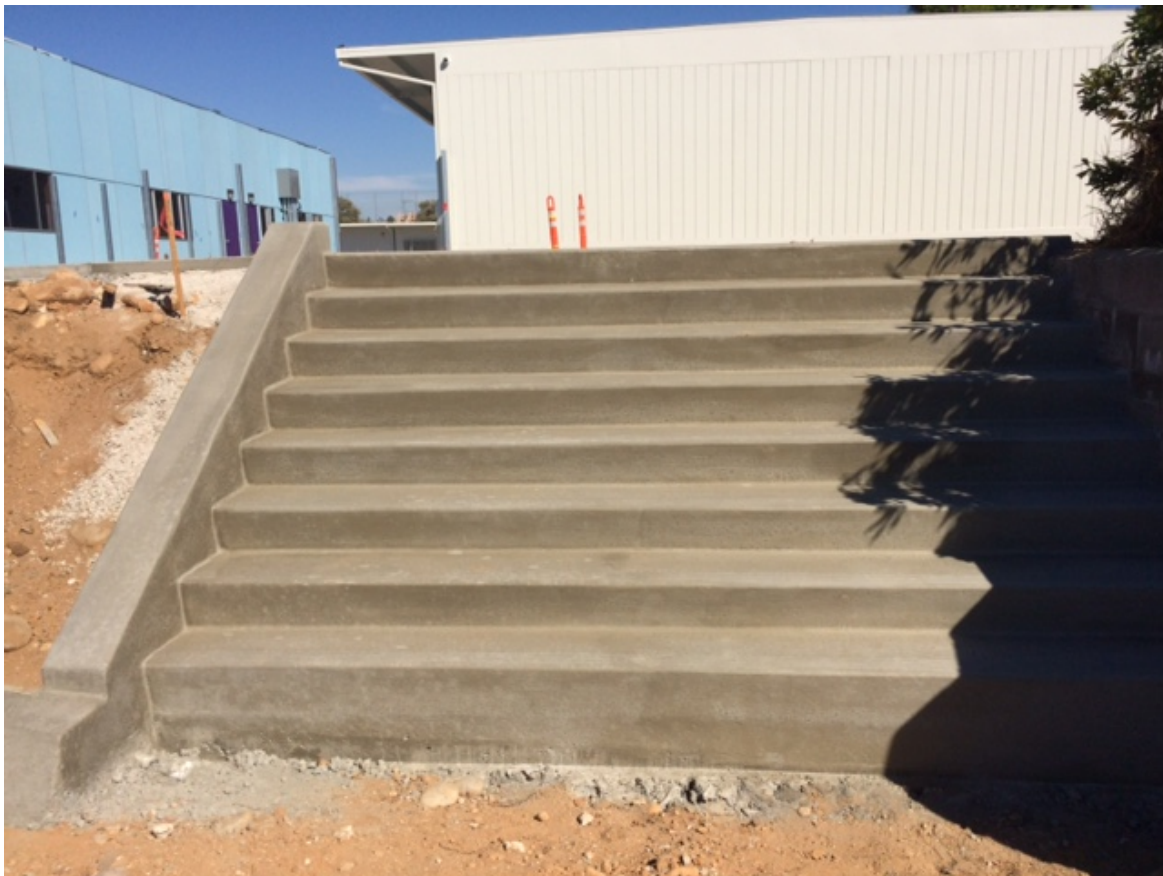
Stairway at front entrance. Admin building in blue.
