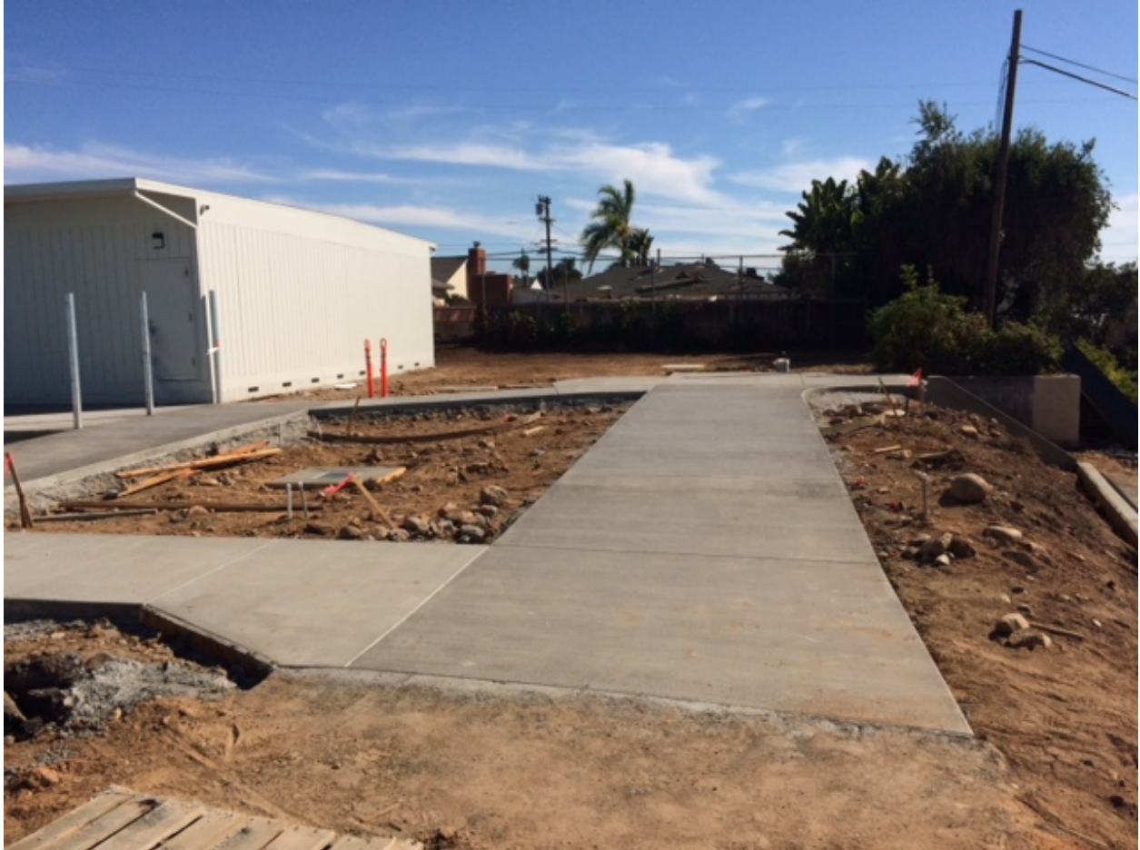
Flatwork and planting beds at front entrance of school. An accessible ramp will be poured in this area.
