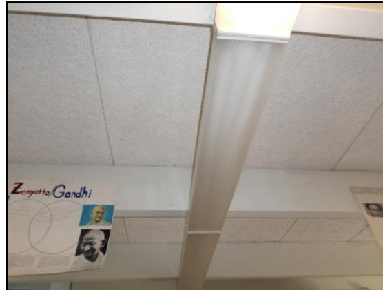
(Item #37) Burned out light bulbs in classroom P32
