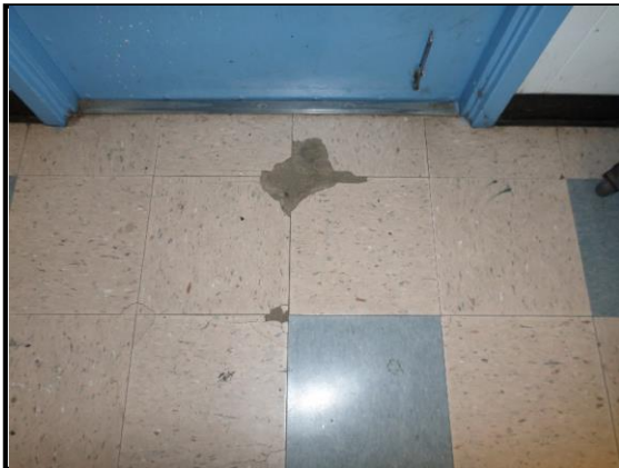
(Item #41) Damaged floor tiles in classroom P32
