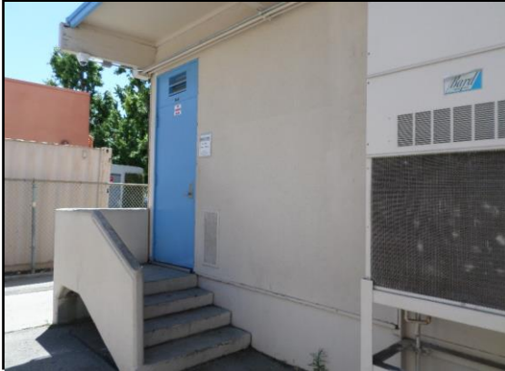
(Item #11) Missing accessible ramp to classroom P33
