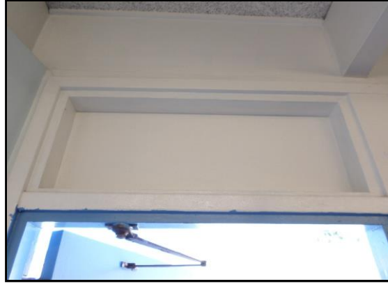
(Item #32) Missing Exit sign in classroom P52
