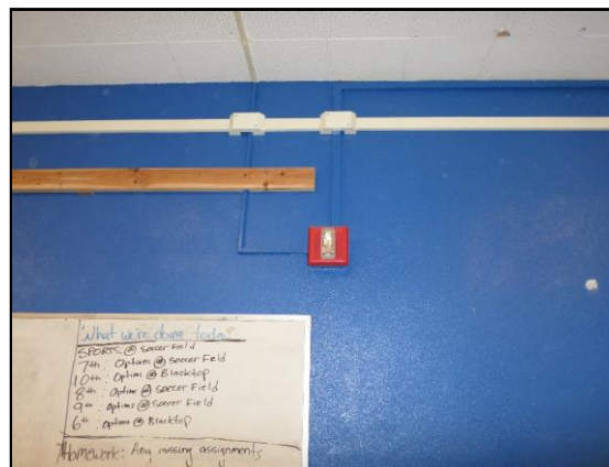
(Item #26) Fire alarm system in classroom
