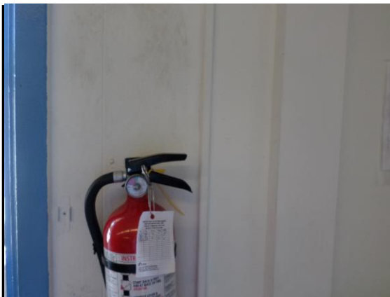
(Item #24) Missing location sign to fire extinguisher
