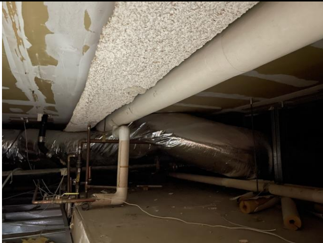
Photo 15: Non-ACM fireproofing on I-Beams above drop ceiling
