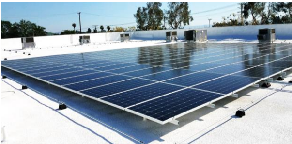
LOCATION Los Angeles, CA STRUCTURE TYPE Rooftop
