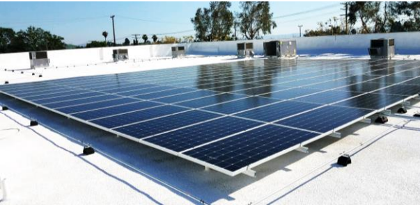
LOCATION Los Angeles, CA STRUCTURE TYPE Rooftop
