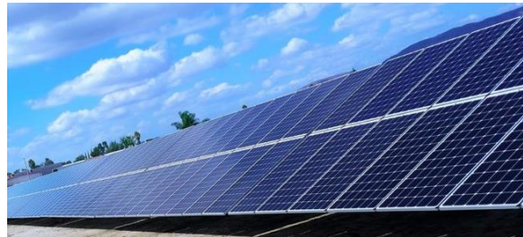
LOCATION San Jacinto, CA STRUCTURE TYPE Ground Mount
