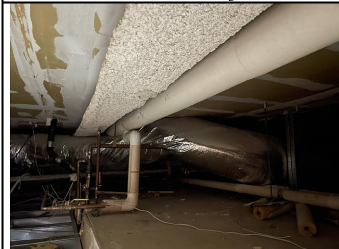
Photo 15: Non-ACM fireproofing on I-Beams above drop ceiling
