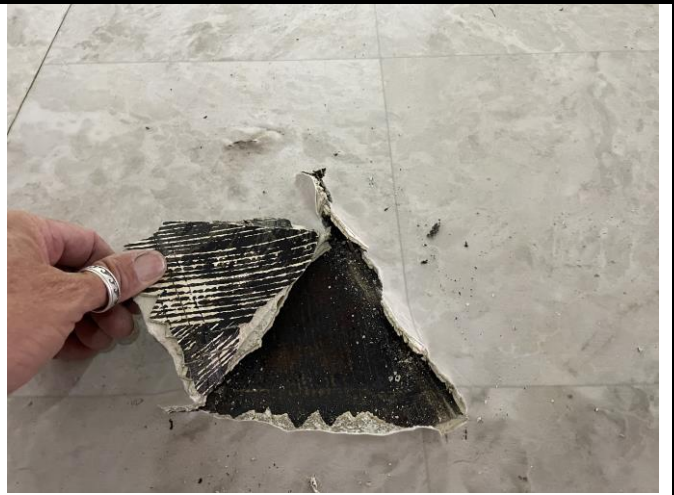
Photo 12: ACM flooring under sheet vinyl
