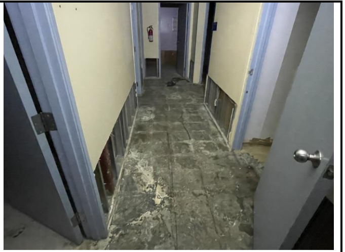
Photo 14: Suite 14 with flooring removed, ACM mastic on slab
