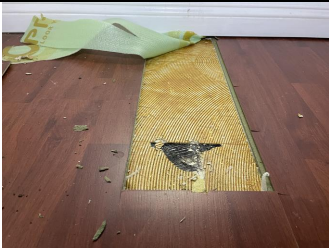
Photo 11: ACM flooring under laminate
