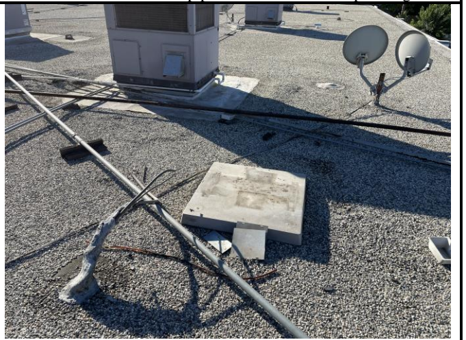
Photo 18: ACM roof mastic at the penetrations and flashings
