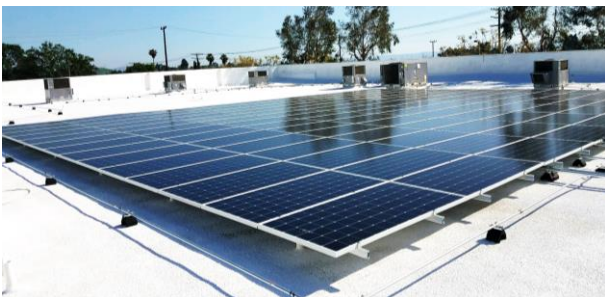
LOCATION Los Angeles, CA STRUCTURE TYPE Rooftop
