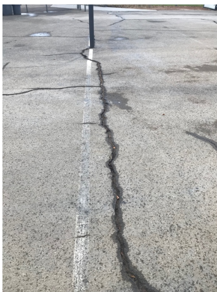
Asphalt at Basketball Court
