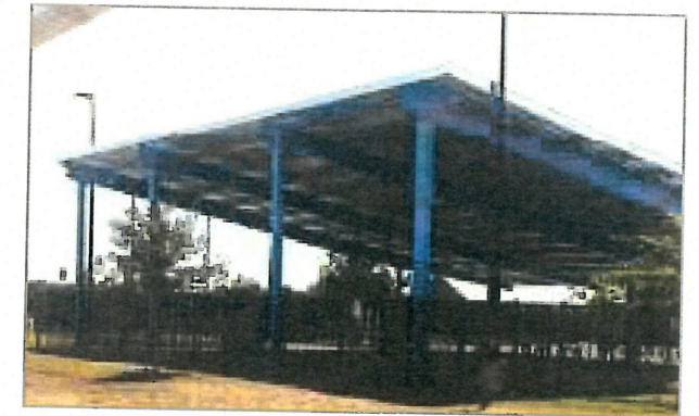
CUSTOM BUILT SHADE STRUCTURE
