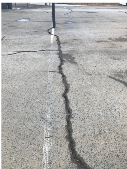
Asphalt at Basketball Court
