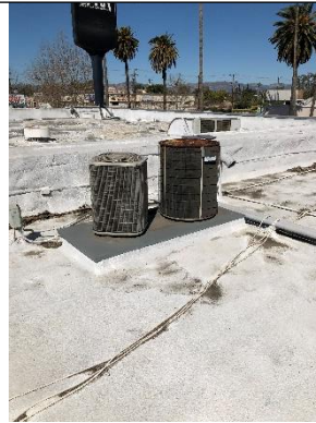
Equipment at Roof
