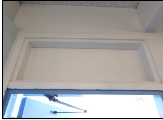
(Item #32) Missing Exit sign in classroom P52
