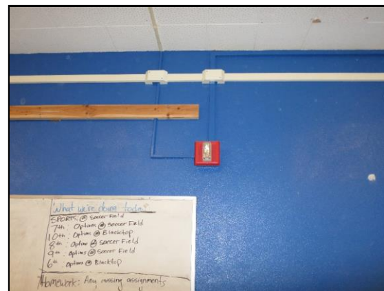
(Item #26) Fire alarm system in classroom
