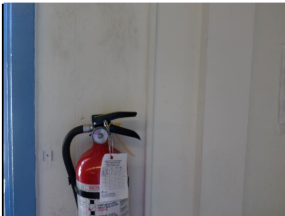
(Item #24) Missing location sign to fire extinguisher
