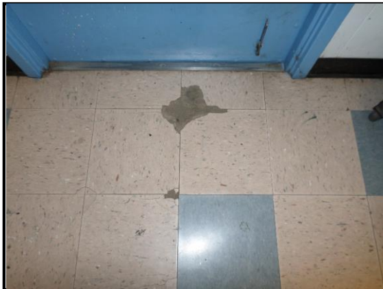
(Item #41) Damaged floor tiles in classroom P32
