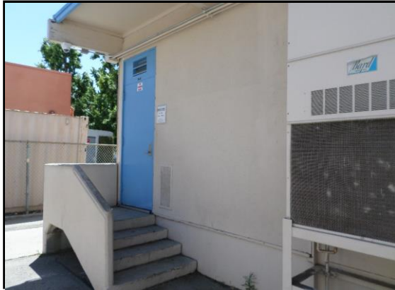
(Item #11) Missing accessible ramp to classroom P33
